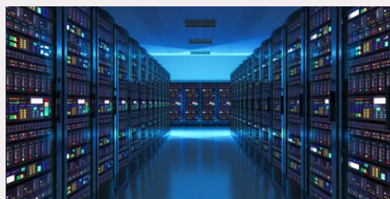
CF Borden Data Center
